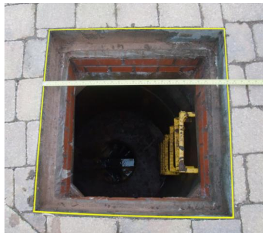
*Incorrect installation and measurement of clear opening
